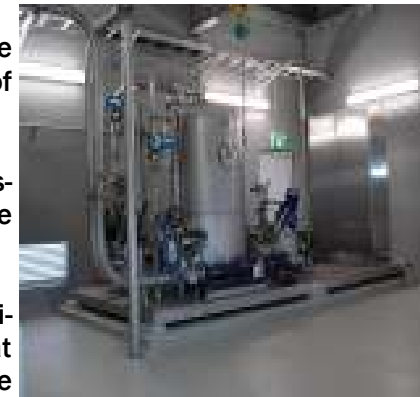
Skid Mounted Crown System Installed at North Shore
