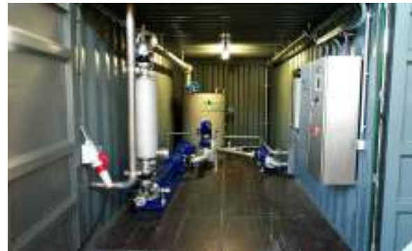
Containerised Crown System Installed at Gifhorn
